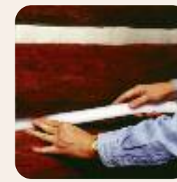
1. Start with logs that are stained with a coating compatible to Log Jam and have properly installed backer material.
