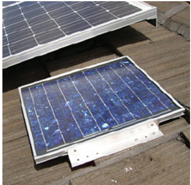
remote solar panel installed on roof
