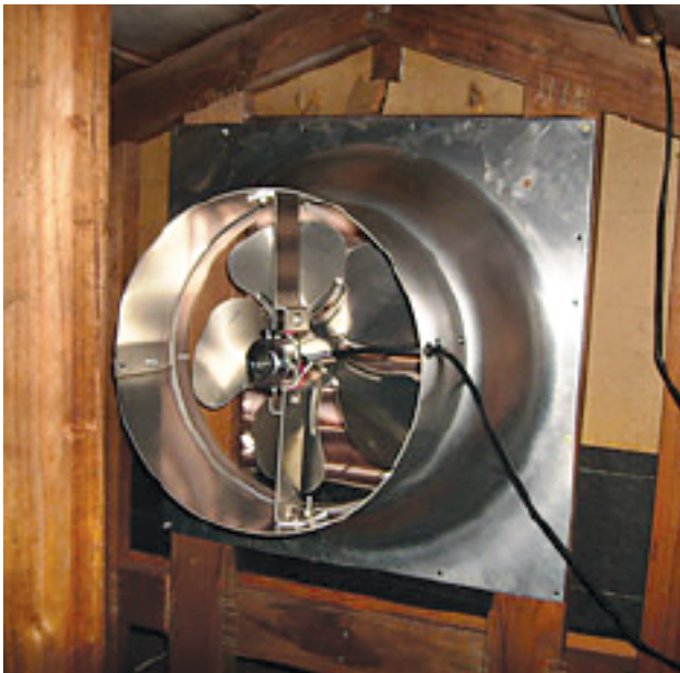
gable mounted fan (view from inside attic)
