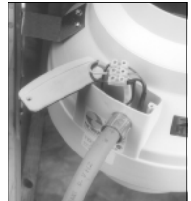
Romex Wiring Top View
