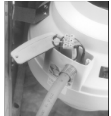
Vista superior, alambrado romex
