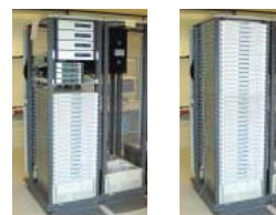
14U for Switches 20U for Servers
