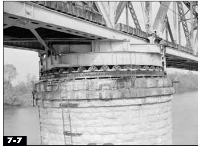
7-7 Large wheels on a track support the weight of a rim-bearing bridge. This bridge (the same as shown in photo 7-1) is supported by forty 20"-diameter wheels on a 25'-diameter track. Historic American Engineering Record; C.N. Beasley
